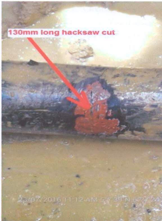
Incident point one (1)
